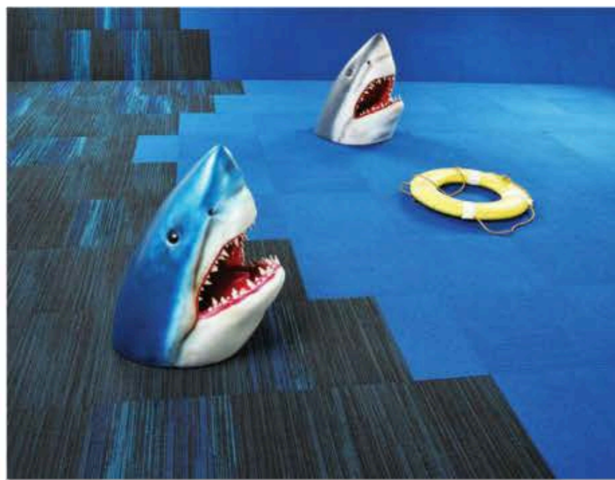
An example of 610 x 610-mm (24 x 24-in.) carpet tiles using the 'quarter-turn' installation method.
